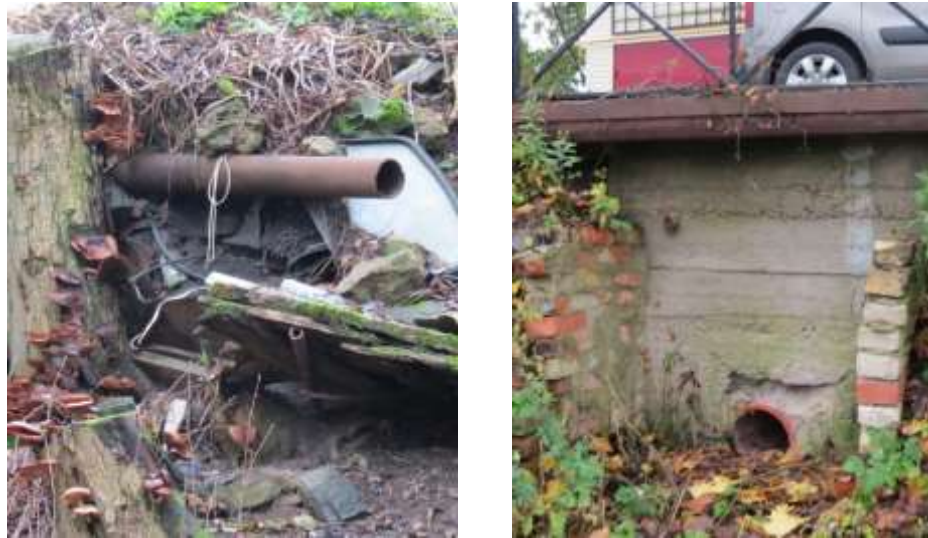
Figure 12. Places of possible illegal sewage flows on the banks of the Setra River (photos by ILRAS).
